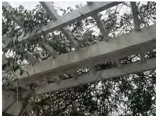
Pergola wood deterioration
