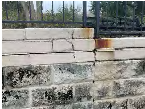
Cracks and settled masonry
