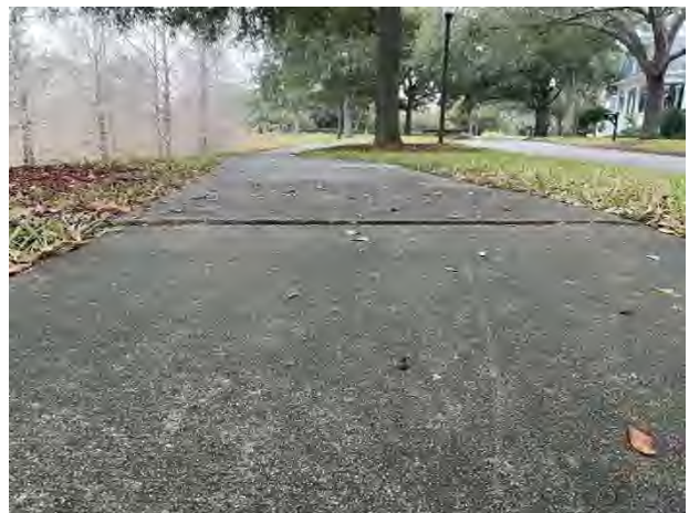
Sidewalk trip hazard
