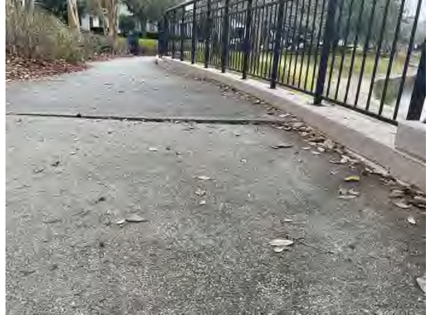
Sidewalk trip hazard
